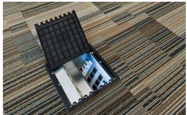
Looking into an electrical box under access flooring.
